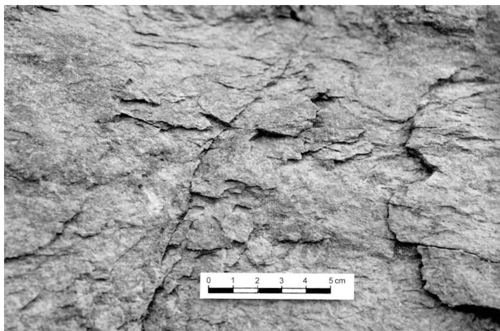
Fig. 11 Weathering form “multiple flakes to crumbling (mF-Pu)”
