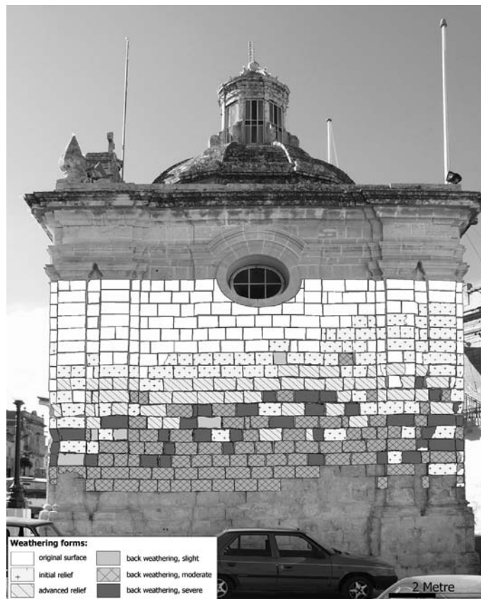
Fig. 4. Mapping of damage forms on the Church of Santa Marija Ta' Cwerra (south façade; 2004) reveals a clear distribution of weathering phenomena. Three zones in vertical order can be distinguished. Severe damage in the form of back-weathering occurs in the area immediately above the plastered lower courses. Further up, the middle zone is seen to have severe to moderate damage. Here alveolar weathering additionally affects numerous building stones. With the exception of a few building stones, the uppermost zone has remained in relatively good condition. These stones have developed a red–brown patina typical of good local building stone. There are, however, areas with organic deposition.
