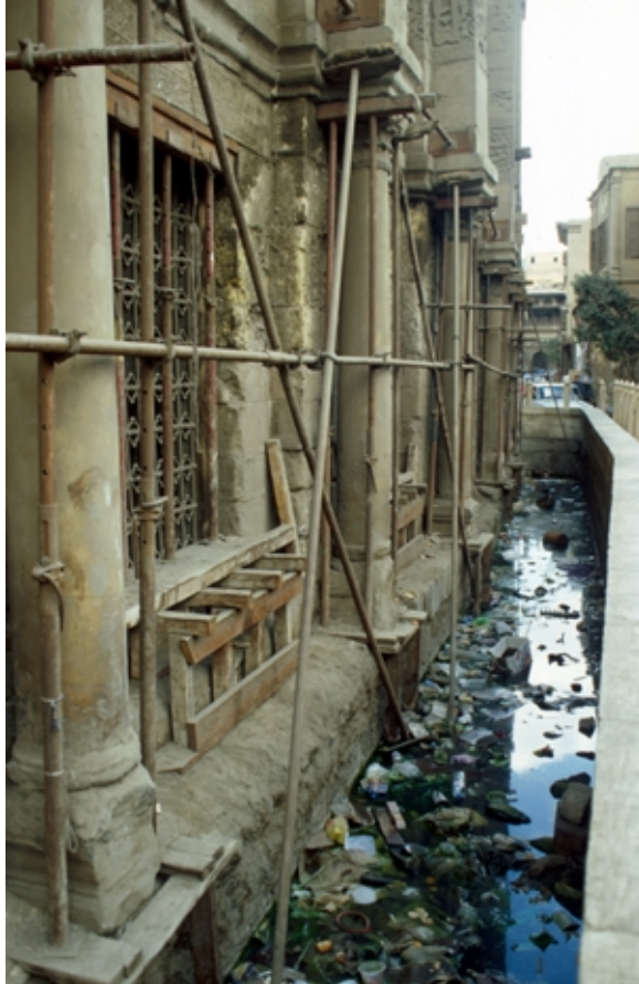
Fig. 7. Weathering damage and elevated water table. Mausoleum of Sultan Al-Mansur Qalawun.
