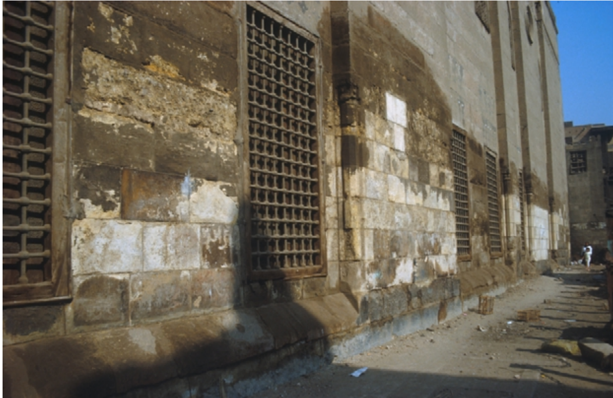
Fig. 6. Weathering damage. Mausoleum of Sultan Al-Mansur Qalawun.
