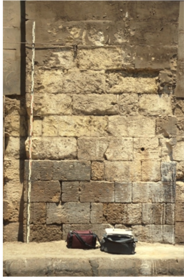
Fig. 5. Weathering damage on a lower part of the El-Merdani Mosque.
